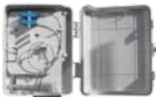
FIBER DISTRIBUTION POINT (AERIAL)
