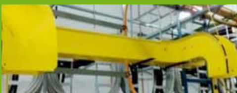
FIBER OPTIC TRUNKING SYSTEM (FOTS)
